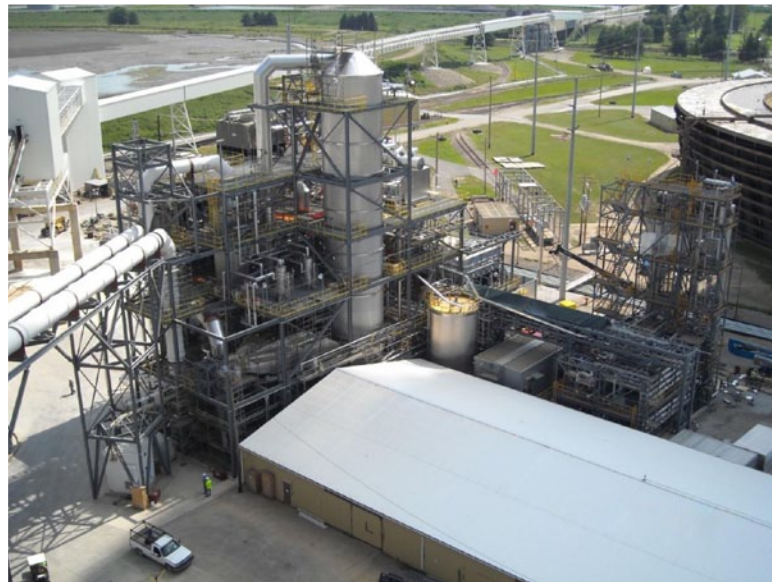
Figure 1. Chilled Ammonia CO 2 Capture Process Validation Facility
