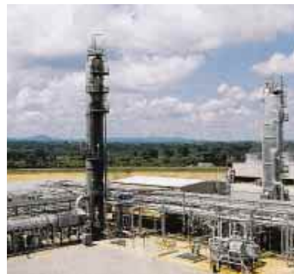
CAPTURE PLANT located in Shady Point, Okla., separates carbon dioxide from its exhaust fumes; the gas is then sold for use in the food industry.
