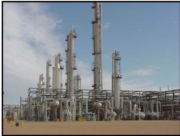
Figure 4.6: Amerada Hess Ryan Holmes Gas Processing Unit, Seminole, TX.
