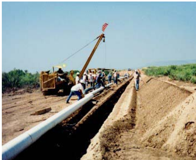
Figure 6.1: Val Verde Pipeline, Petro Source Carbon Company, cited October 11, 2002 at http://www.petrosourcecorp.com/HP_co2.htm
